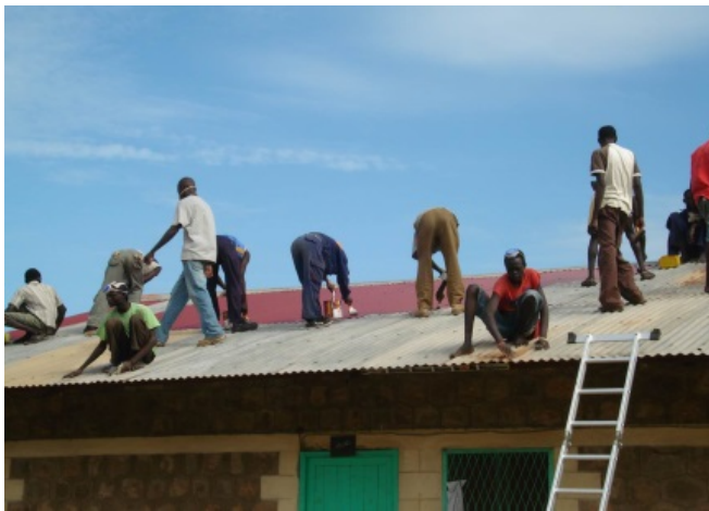
Youth engaged in renovation of Juba Youth centre: an activity carried out by UNOPS using the on-the-job training approach in 2010
